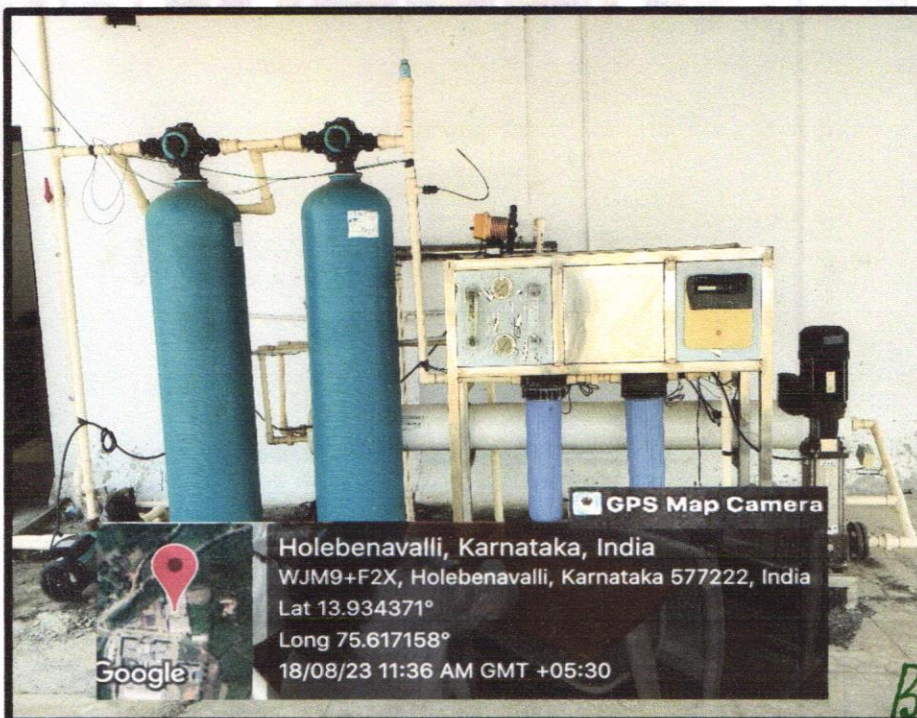
SEEWAGE TREATMENT PLANT (STP)
