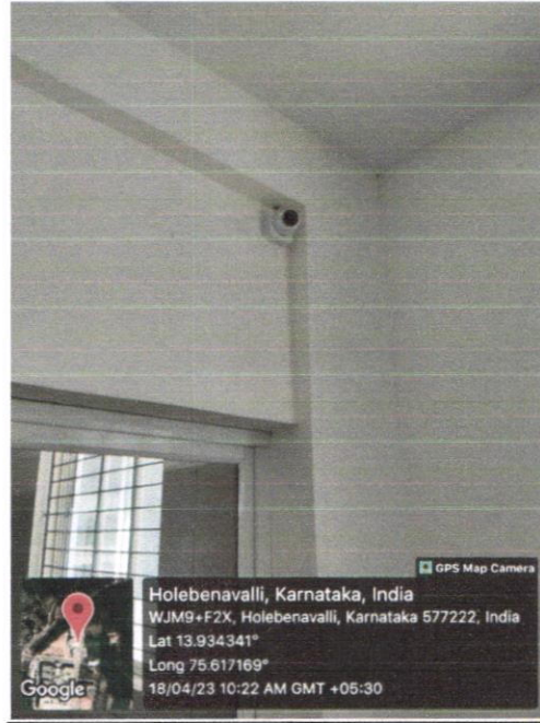
GIRL'S COMMON ROOM AREA WITH CCTVCAMERA
